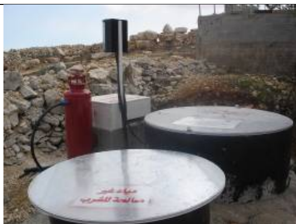
Photo 2: the installed wastewater Treatment Plant at Mousa Mohammad Hasasnah's House - Ash Shuyukh Village - Hebron Governorate
